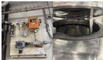
Control oxygen levels below 5vol.% to minimize fire and explosion risks
