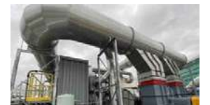
Zeolite wheel + regenerative thermal oxidation furnace (RTO)
