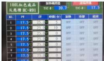
PLC-HMI system with timing and temperature control functions, promptly initiating escape procedures and alarms
