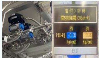
PLC-controlled system with automatic pressure release and simultaneous opening of vacuum and exhaust valves in case of excessive pressure
