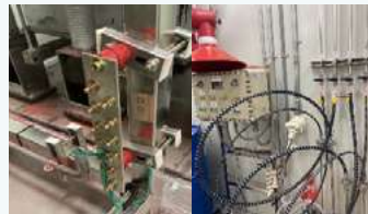
Decrease fire and explosion risks by implementing anti-static and grounding devices
