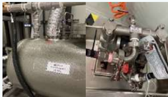
Reduce dispersion risk by transporting liquid raw materials through pipelines
